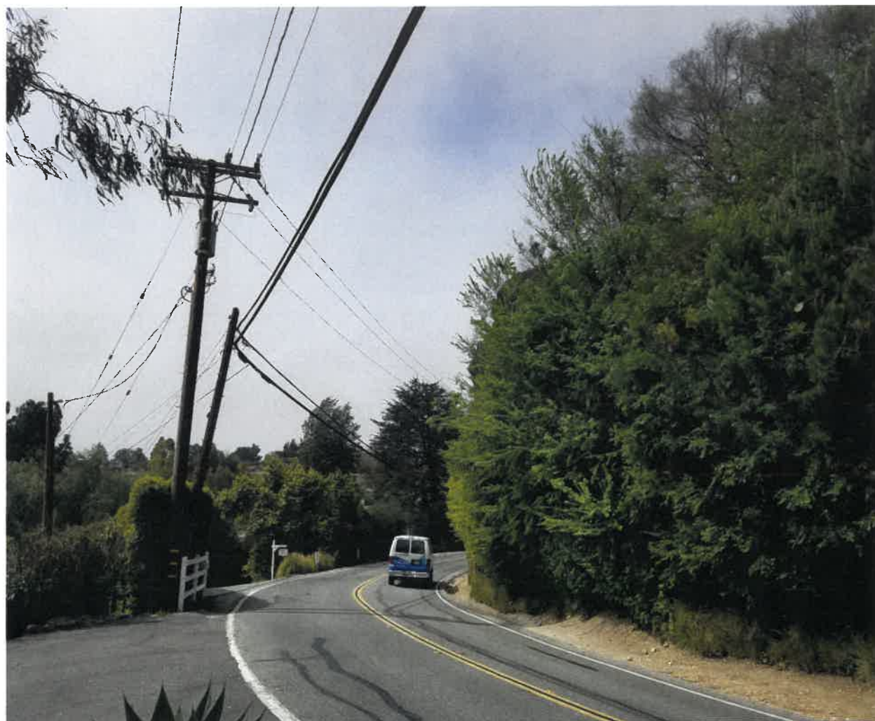
Existing Utility Lines on Eastfield Drive (2019)
