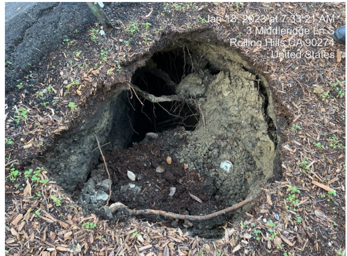
Photo 4 - Closest sink hole to catch basin was about 3' in diameter and about 8' deep (bottom of SD).
