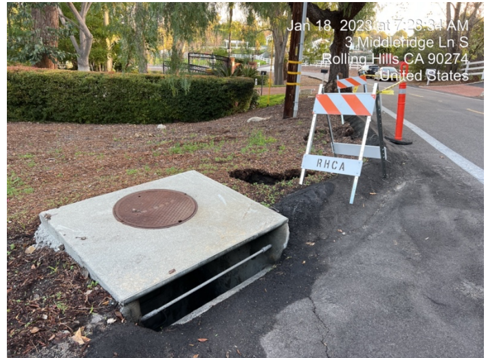
Photo 2 - (2) Sink holes were within 16 LF n/o catch basin at STA 7+84.
