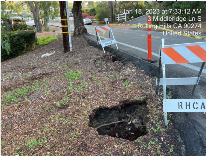
Photo 3 - Sink holes were outside of the roadway and behind AC rolled curb.
