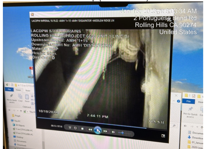
Photo 6 - Video clips were reviewed to determine length of corroded CMP from station to station.
