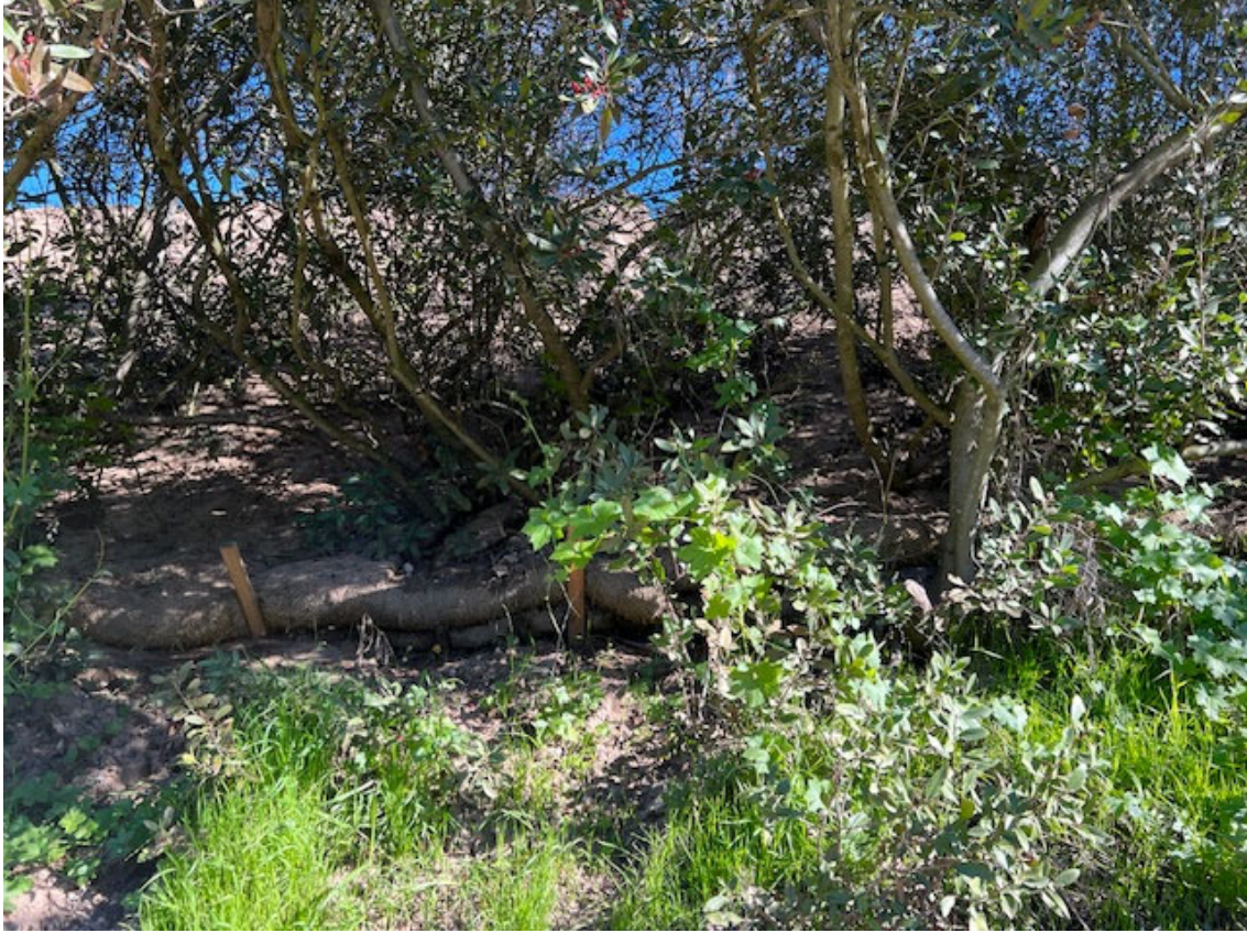
Top: Path of runoff eroding onto Johns Canyon Trail (2/7/23)
