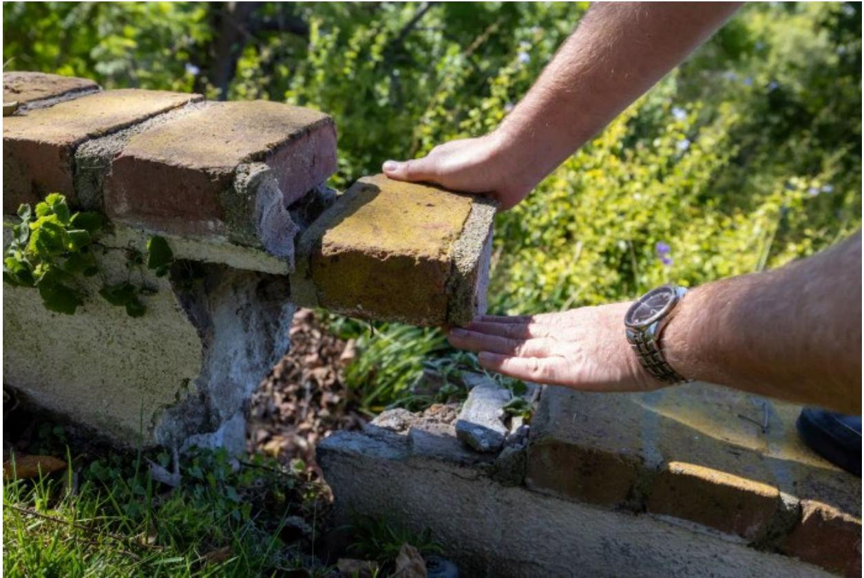
Figure 6: September 30, 2024 Crack running through retaining wall
