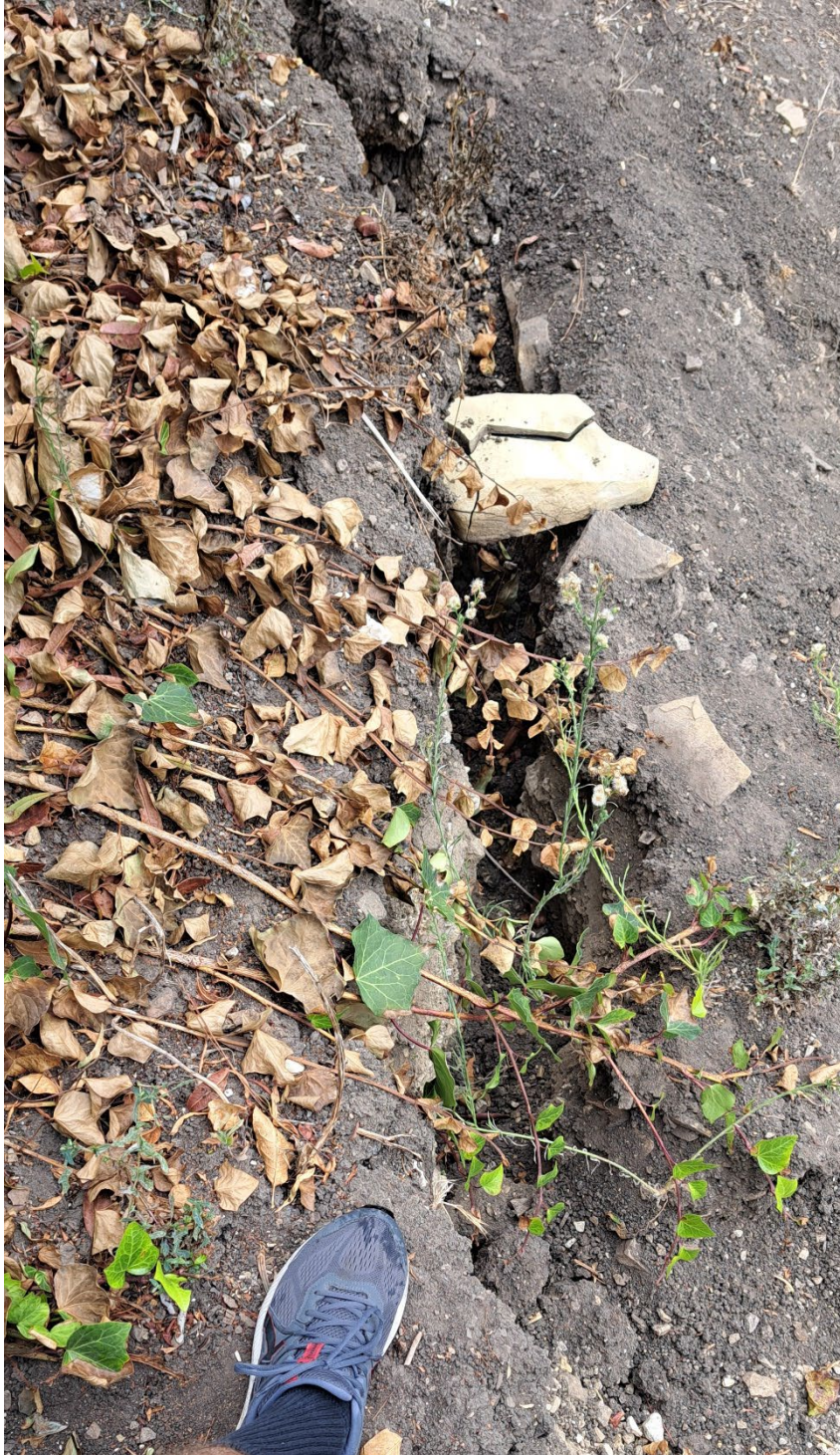
Figure 3: September 24th, 2024 Showing Expanding Crack and vertical movement
