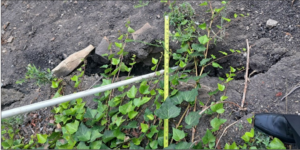
Figure 1: September 9, 2024 Crack between 3 and 5 Quail Ridge Rd. S.
