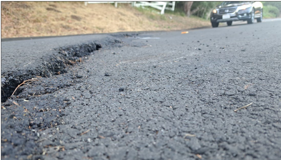
Figure 2: September 9, 2024 Crack and movement on Quail Ridge Rd. S.
