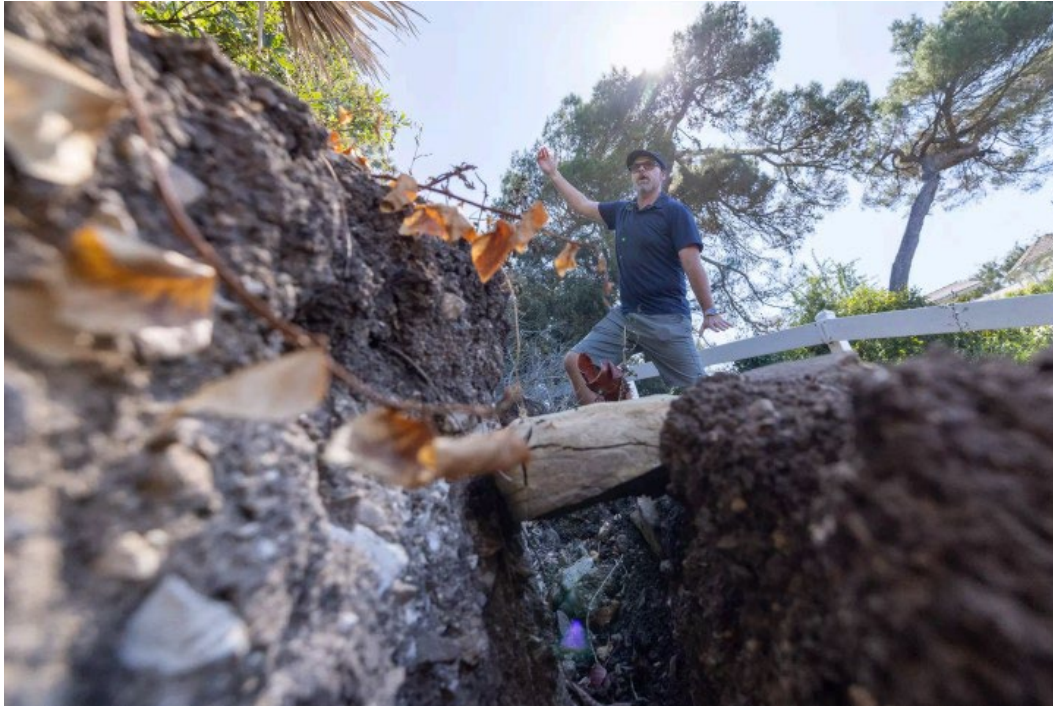
Figure 4: September 29, 2024 showing crack widening and vertical movement
