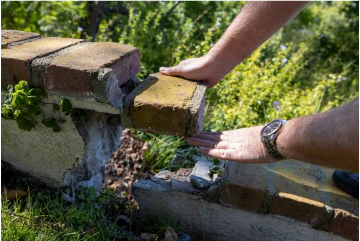
Figure 6: September 30, 2024 Crack running through retaining wall
