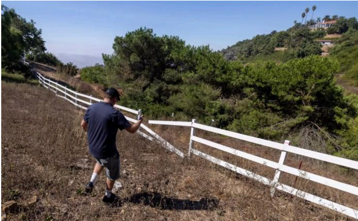
Figure 5: September 29, 2024 showing crack all the way through property and damaging fence
