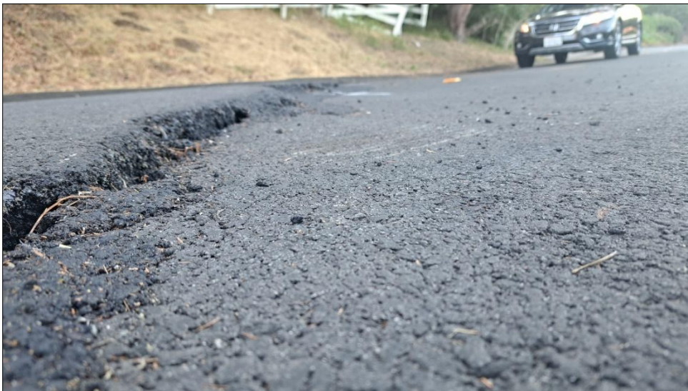
Figure 8: September 9, 2024 Crack and movement on Quail Ridge Rd. S.
