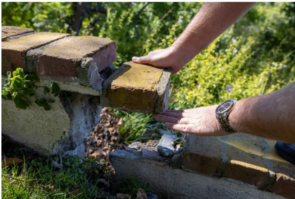
Figure 12: September 30, 2024 Crack running through retaining wall
