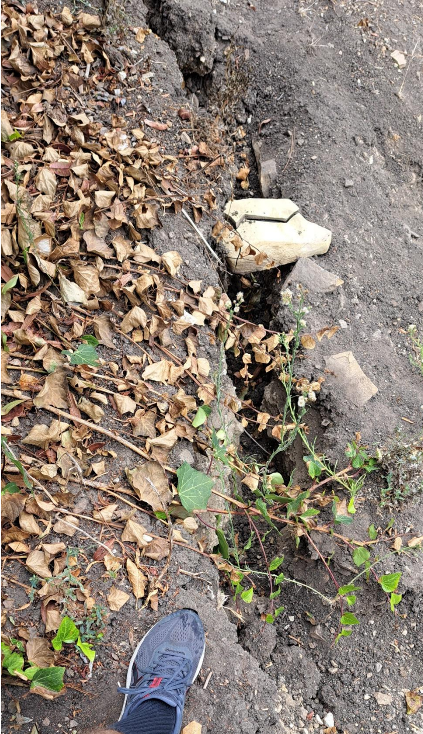
Figure 9: September 24th, 2024 Showing Expanding Crack and vertical movement
