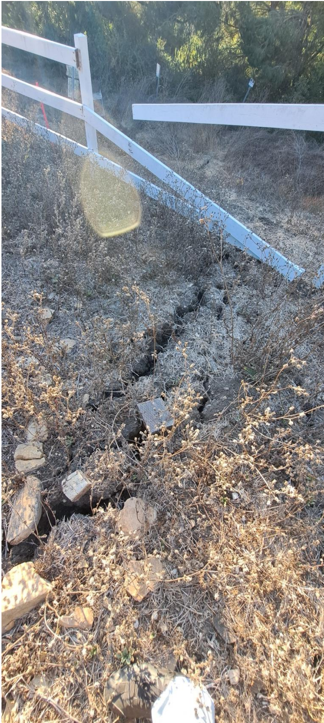
Figure 4: November 11, 2024 Canyon Below 3 Quail Ridge S - Increased Fence Damage
