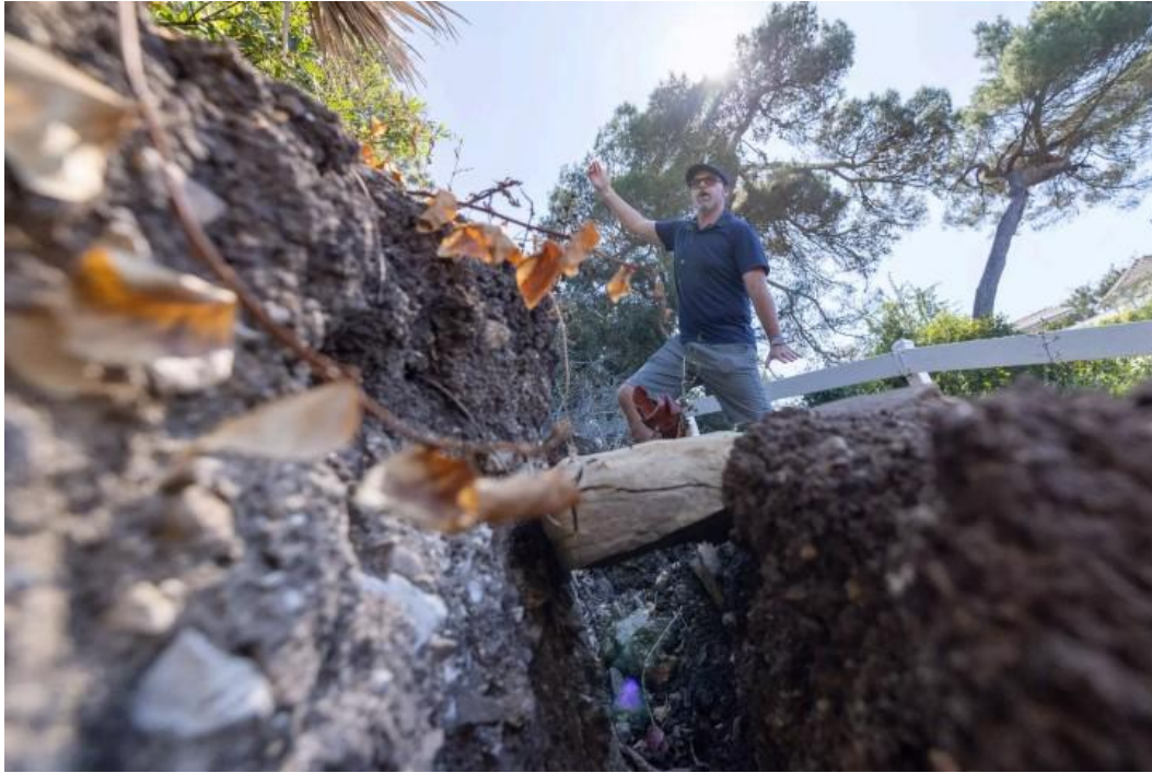
Figure 10: September 29, 2024 showing crack widening and vertical movement
